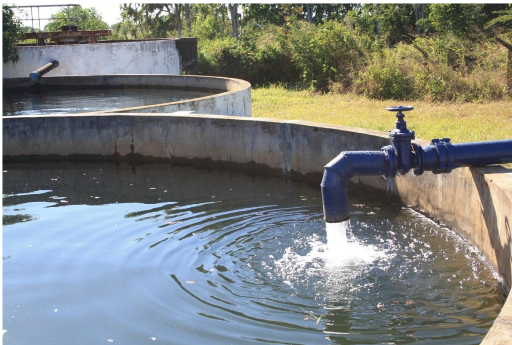
Figure 3-6 : Águas de Chimoio drinking water treatment plant in Chimoio.
