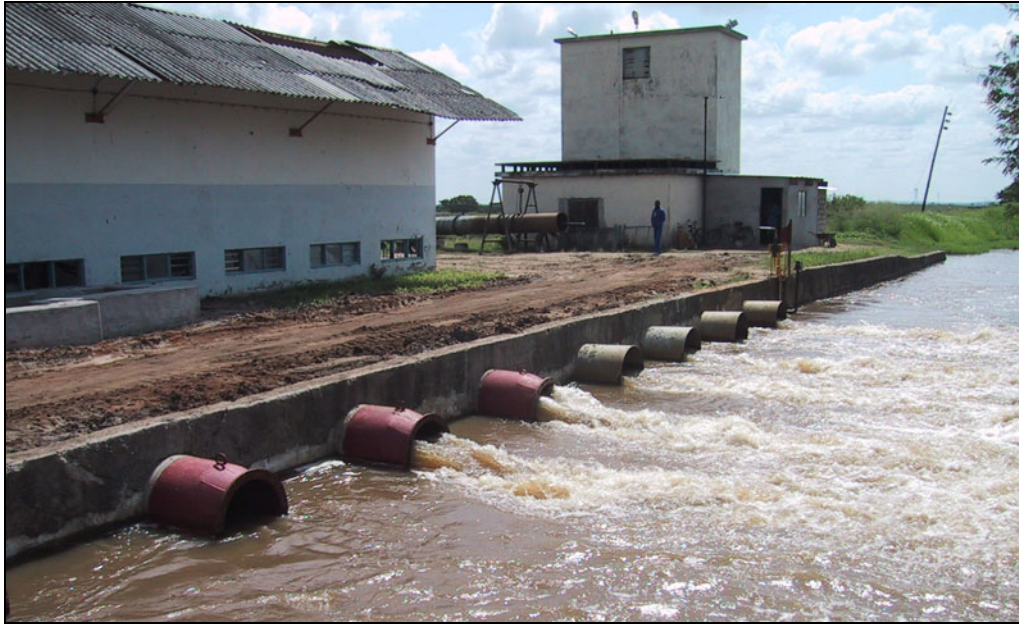
The intake and pumping station of Mafambisse Sugar Estate is the largest hydraulic installation in the Pungwe River
