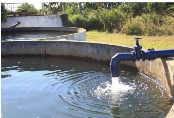
Figure 3-2 : Aguas de Chimoio drinking water treatment plant in Chimoio.
