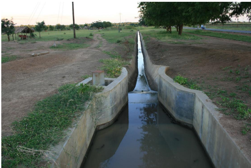
Figure 13 Recording flow in an irrigation scheme, Zimbabwe
