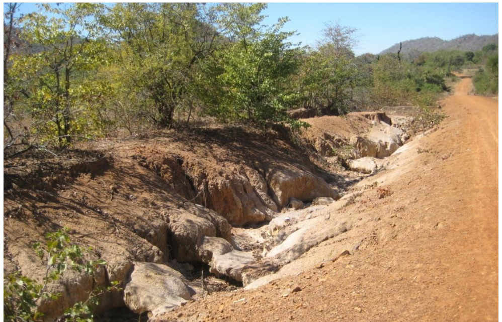
Figure 44 Gullies at Manjarenji Dam
